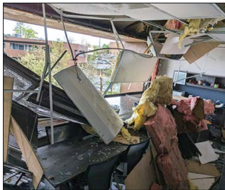
AFTER THE STORM. A view inside FTN's offices following the tornado that struck Little Rock March 31.
