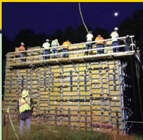
Water Treatment and Intake Facilities Exp. Clarksville Light & Water Company
